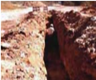
Worker in a trench with no protective system, it's also not sloped or benched and has no means of egress.
