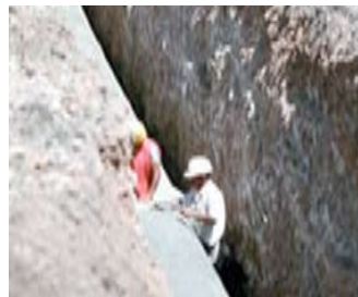
Not protected from cave-in, nor does there seem to be safe access or egress from the trench
